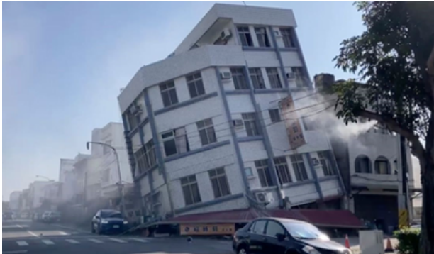
A partially collapsed building following the quake in Hualien, eastern Taiwan, on Wednesday. Image Source: TVBS/AP
