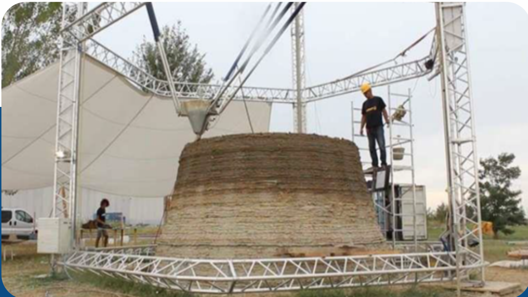
Figure 1: WASP low-cost material shelter | Source:
